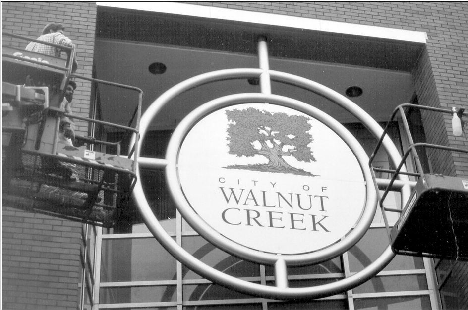
FINISHING TOUCH — Workers installed the official City emblem on the North Broadway side of the new City Hall/Police addition on Nov. 15.
