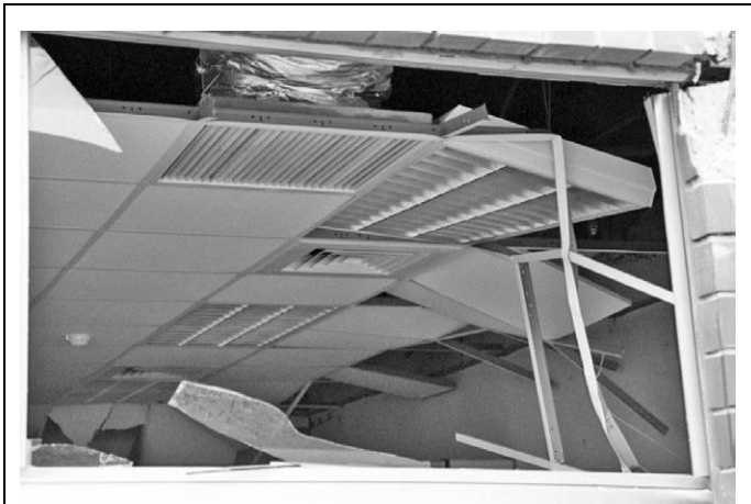
FIGURE 1 Damaged Ceiling System
