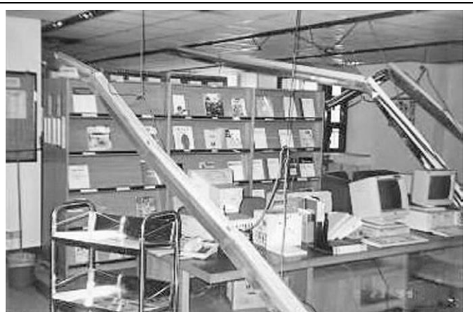
FIGURE 2 Collapsed Light Fixtures
